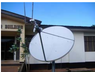
1.8m VSAT Terminal Outdoor Dish & RF
